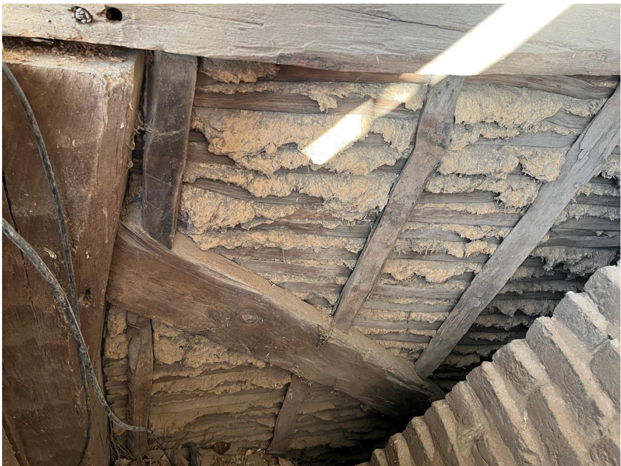
Site Photo 5. Evidence by chimney of lathe and plaster.
