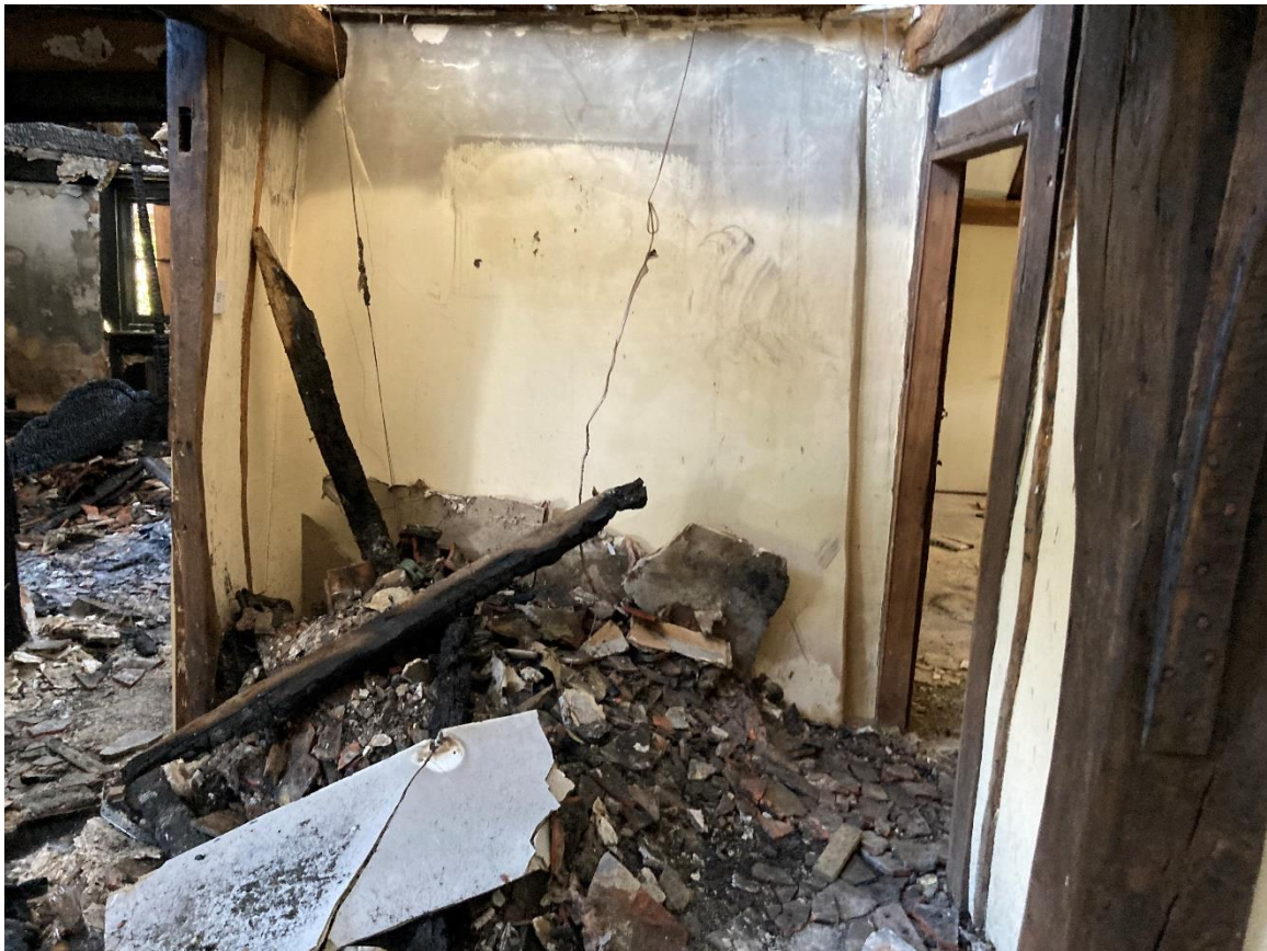
Site photo 15. Area of ground floor with fire damage (Looking west)
