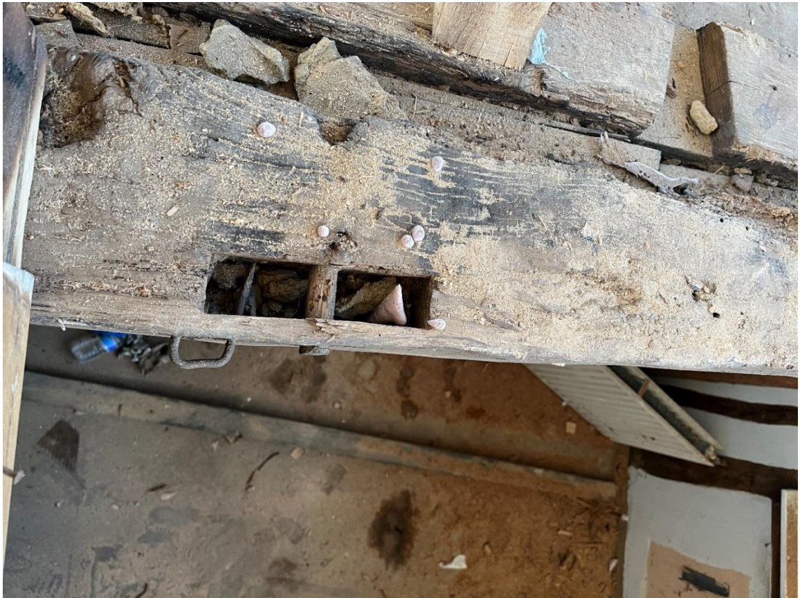
Site Photo 8. Showing historical staples
